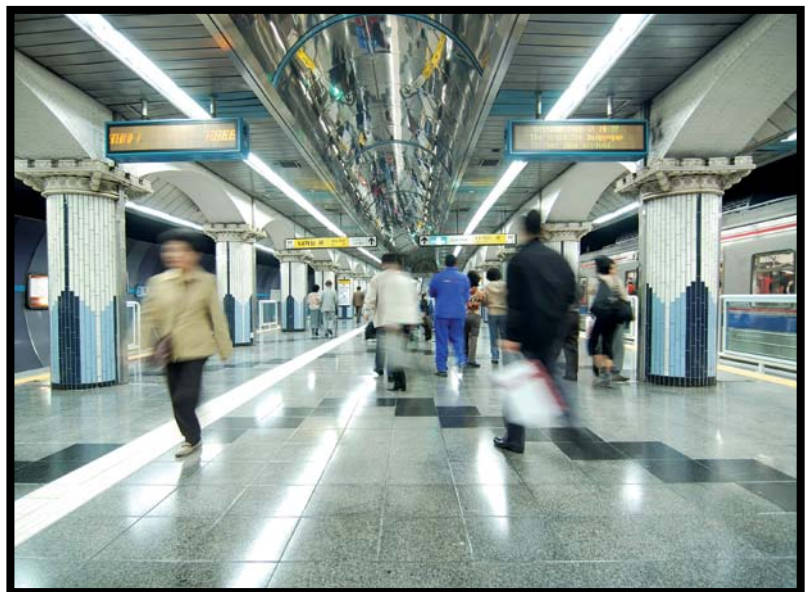
COE equipment will be responsible for the transmission and management of over 8000 cameras across Lines 1, 3 & 4 of Seoul's Metro network.
